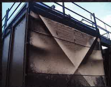
Willowcreek Church Marley Cooling Tower
