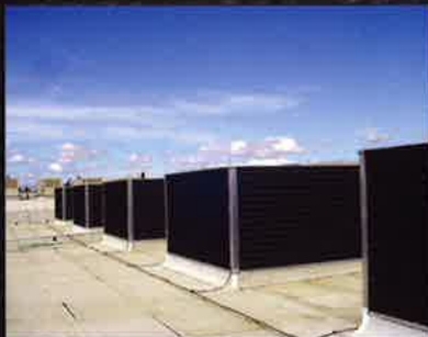
Office Building Rooftop Economizers
