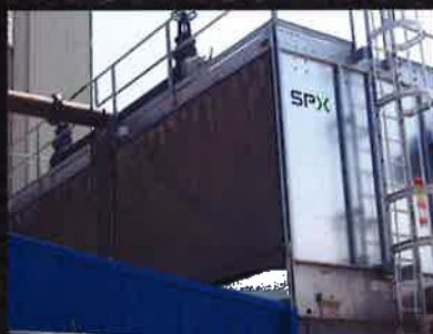
Glass Processing Plant Cooling Towers
