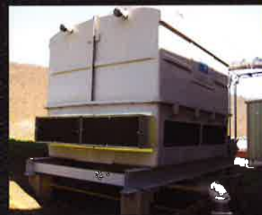
Osram Sylvania Plant Thermal Care Cooling Tower
