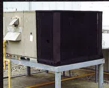
Physics Laboratories HVACR Equipment
