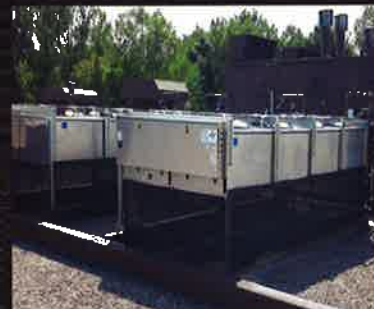
Grocery Store Chain Rooftop Condensing Units
