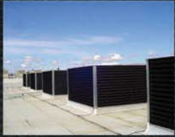
Office Building Rooftop Economizers
